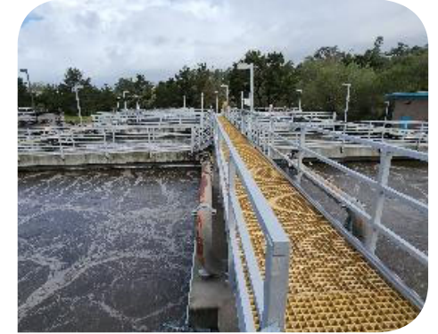
Cambria CSD WWTP
